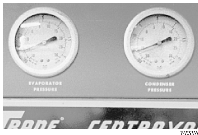
Fig. 2 Evaporator and condenser gauges These tell you immediately whether the machine has the minimum amount of refrigerant for efficient operation. They do not tell you the actual amount. The condenser pressure provides an uncertain indication of excessive charge.
